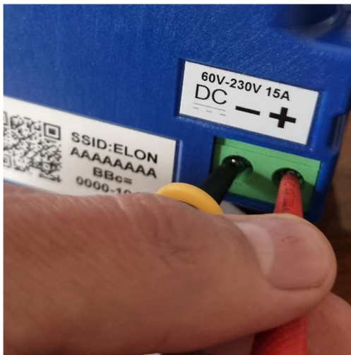
Figure A1 Checking DC voltage
