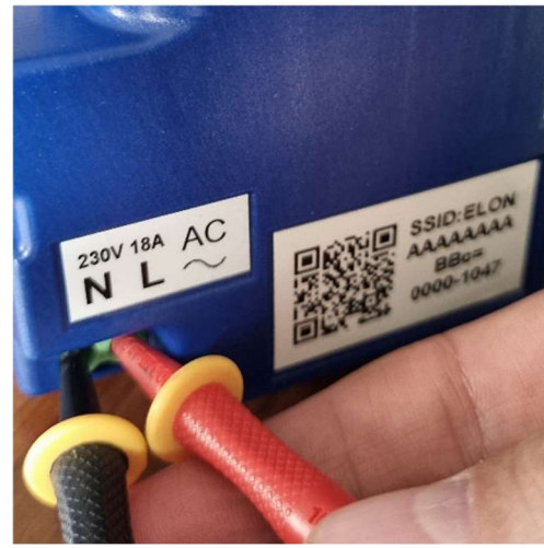
Figure A2 Checking AC voltage
